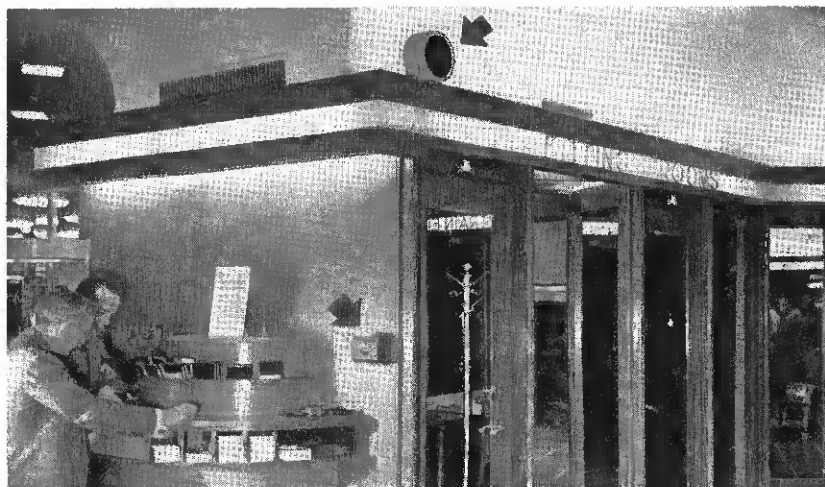
TYPICAL REMOTE —Switchbox and 8-inch p.m. speaker serves the fitting room
